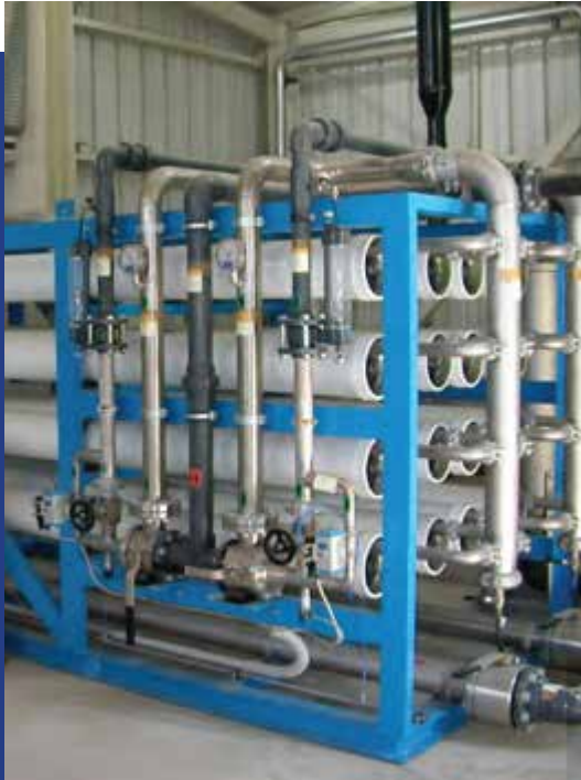
Spiral membrane Reverse Osmosis system
