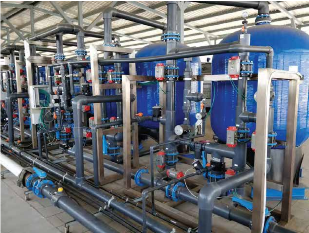
Pressure sand filters (PSF) + Activated Carbon Filters (ACF) + Softeners & De-mineralisers
